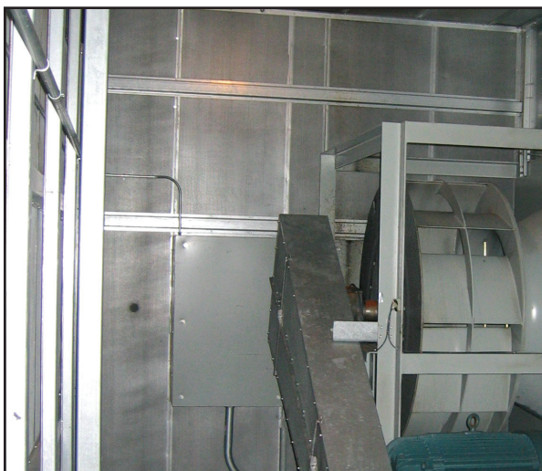
AHU Plenum Interior
