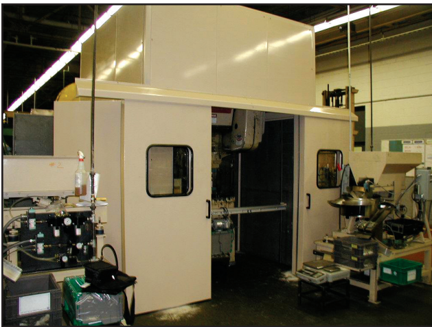
In-Plant Equipment Building
