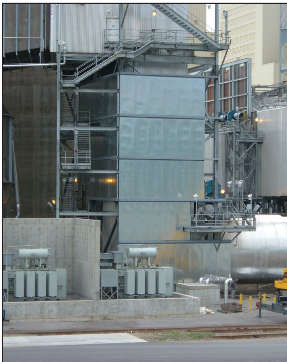
Utilities Barrier Wall
