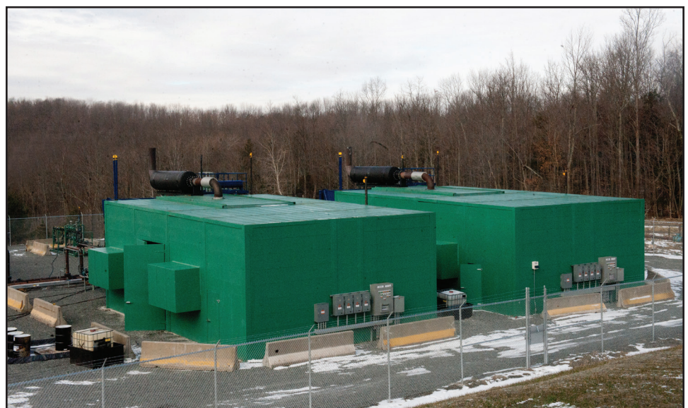
Midstream Compressor Buildings
