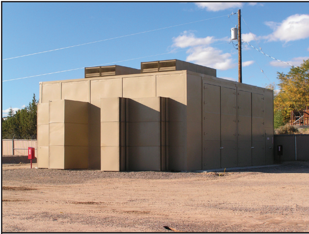
Dual Midstream Compressor Building
