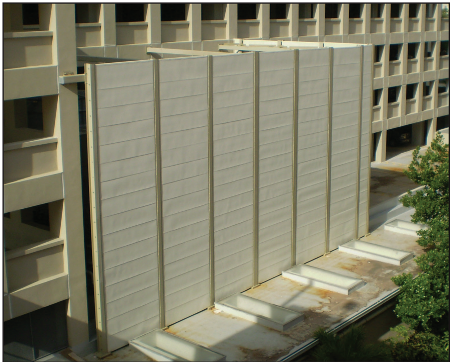
Cooling Tower Barrier Wall System
