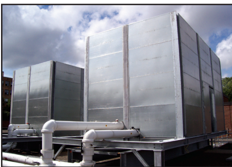
Roof Top Chiller Barrier Wall
