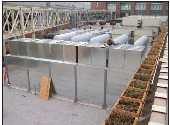
Multiple Generator Enclosure
