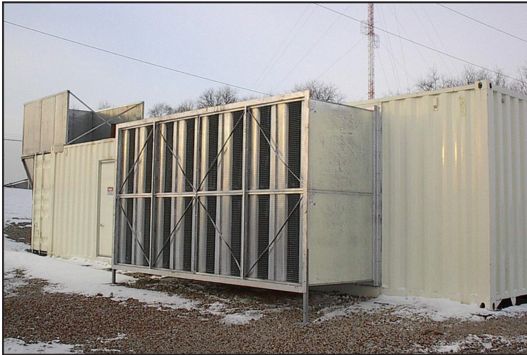
Generator Enclosure Ventilation Silencers
