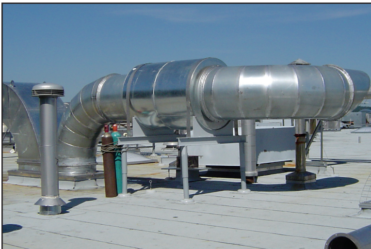
Roof Top Factory Exhaust Silencer
