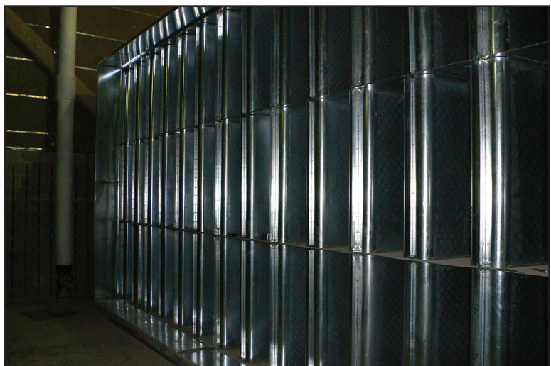
Generator Room Intake Silencer Bank
