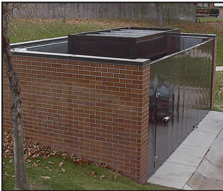
Chiller Barrier Wall
