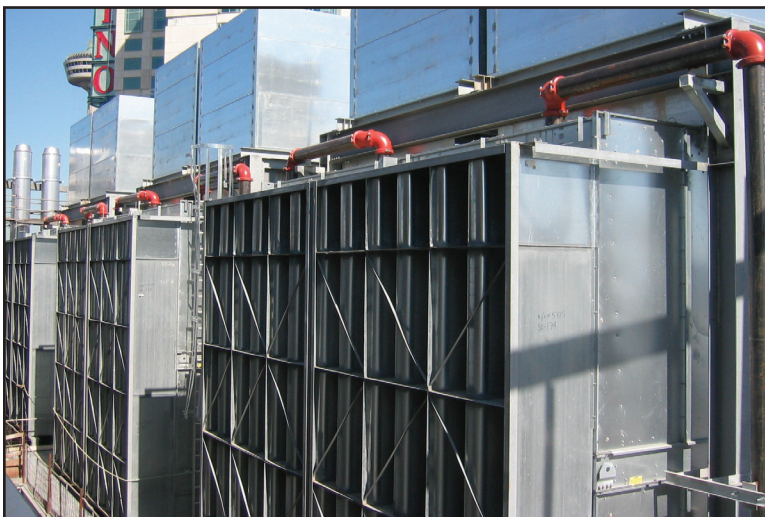
Cooling Tower Inlet and Discharge Silencers
