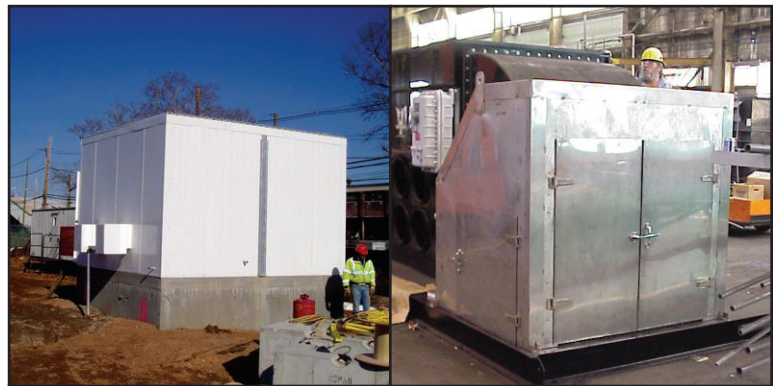
Air Compressor Enclosure
