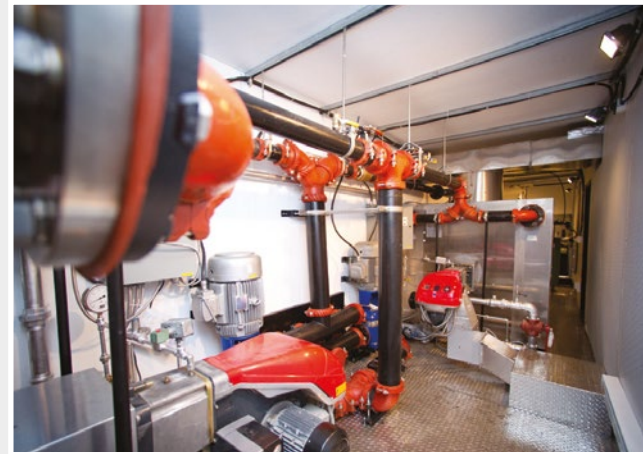
Two 8 million Btu/hr all stainless steel high efficiency condensing boilers with fully modulating burners
