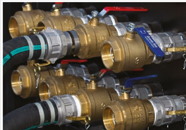
Supply and return manifolds with customized connections and cam lock fittings for quick and easy setup / takedown
