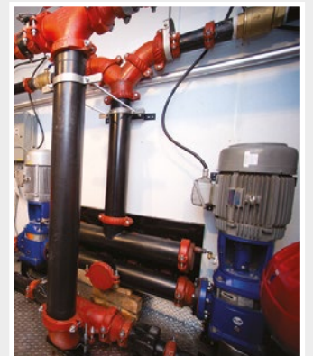
Equipped with 2 sets of pumps providing 100% redundancy
