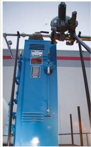
ASME propane vapourizer for boiler and the generating set fuel supply
